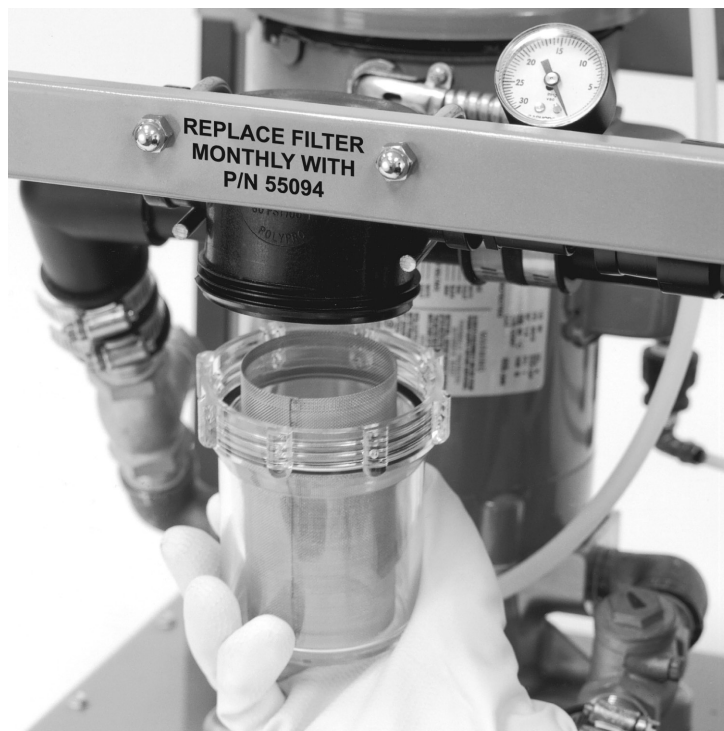
Figure 12. Intake Solids Collector Location
